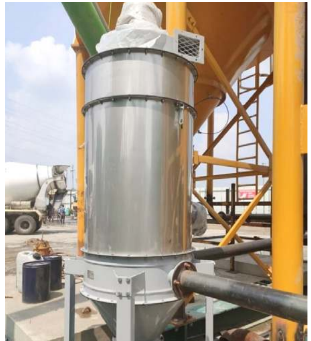
Ground Mounted Dust Collector
